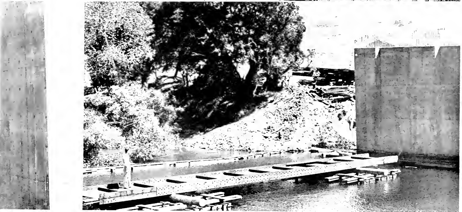
At top—Existing narrow bridge across Pajaro River. Center—Three wide concrete piers ready for steel erection. At bottom—Large steel girder floated into position on rafts preparatory to raising with power crane
